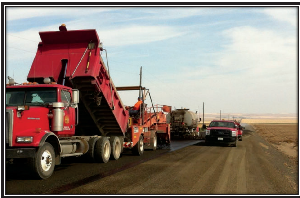
Grant County Road Crew shooting the prime or penetration shot of HFE-150 on the last phase of R-NE between Wilson Creek and Hartline.
