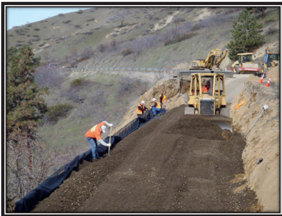
Chelan County Road Crew building an MSE wall on North Dryden Road near Dryden. The project's goal was to stabilize a chronically unstable roadway embankment.
