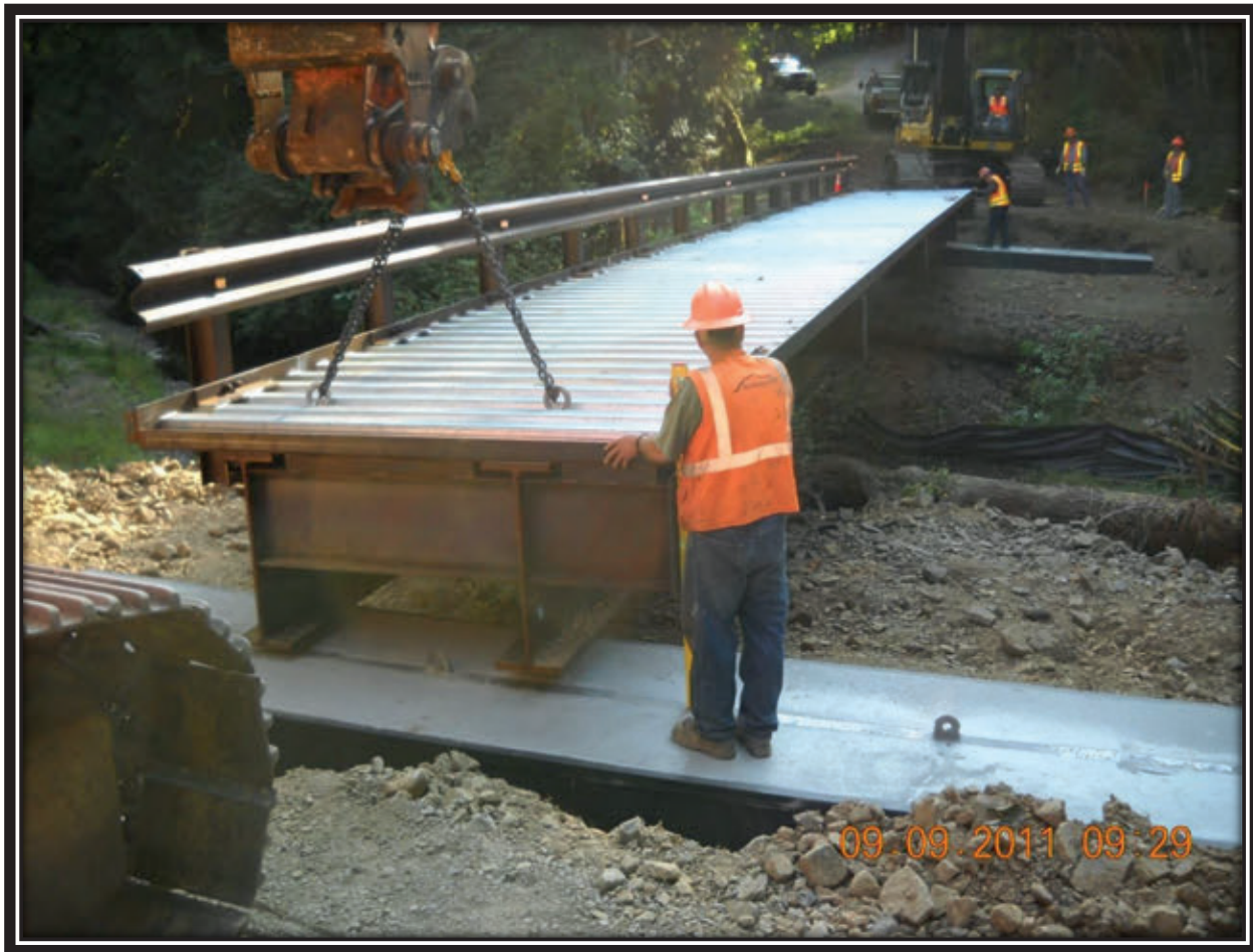
Cowlitz County Road Crew installing a modular steel emergency access bridge intended to provide alternate access during flooding that frequently closes Ostrander Road.
