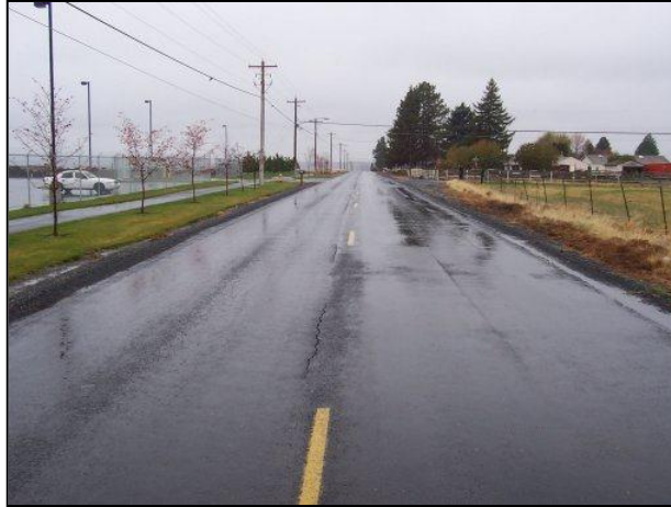
Before improvement, narrow and breaking down.
