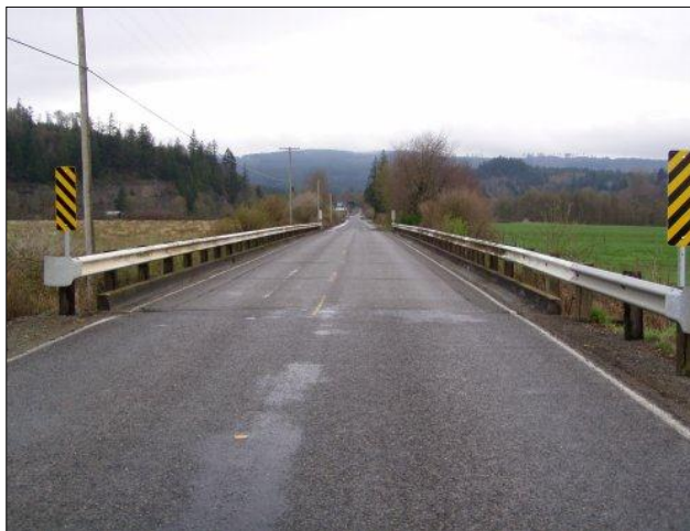
The old bridge was deficient in other ways.
