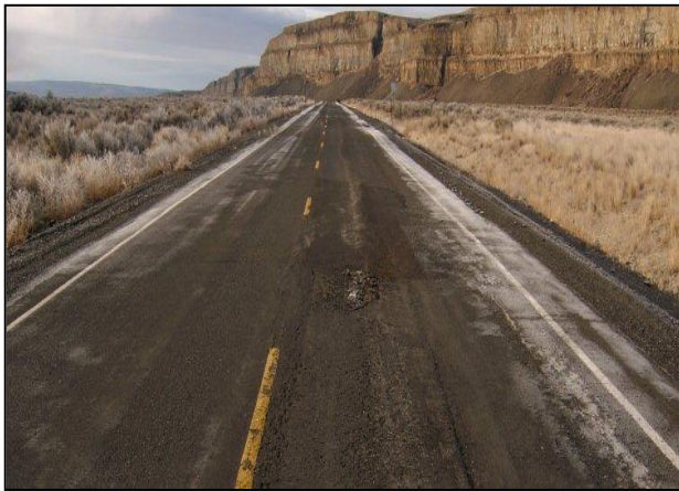
The old surface: rutted, worn, and dangerous.
