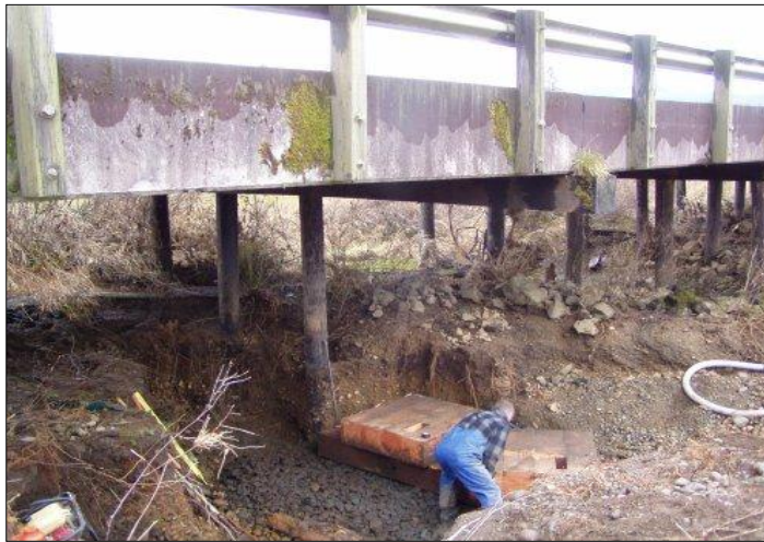
The old structure sustained serious pile damage.
