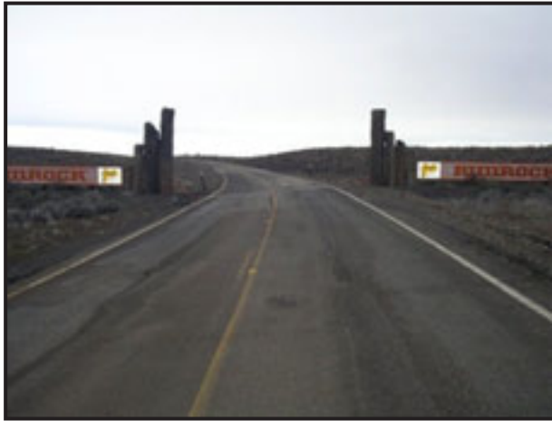
Failing surface conditions on Coulee Meadows.
