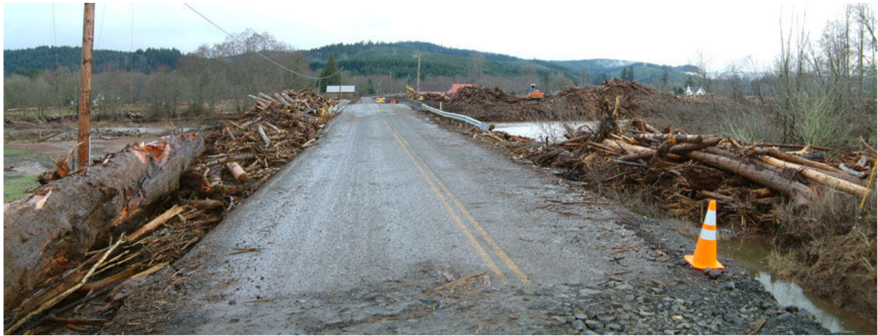
Lewis County's Stillman Creek Bridge during the recovery phase of flood fight.
