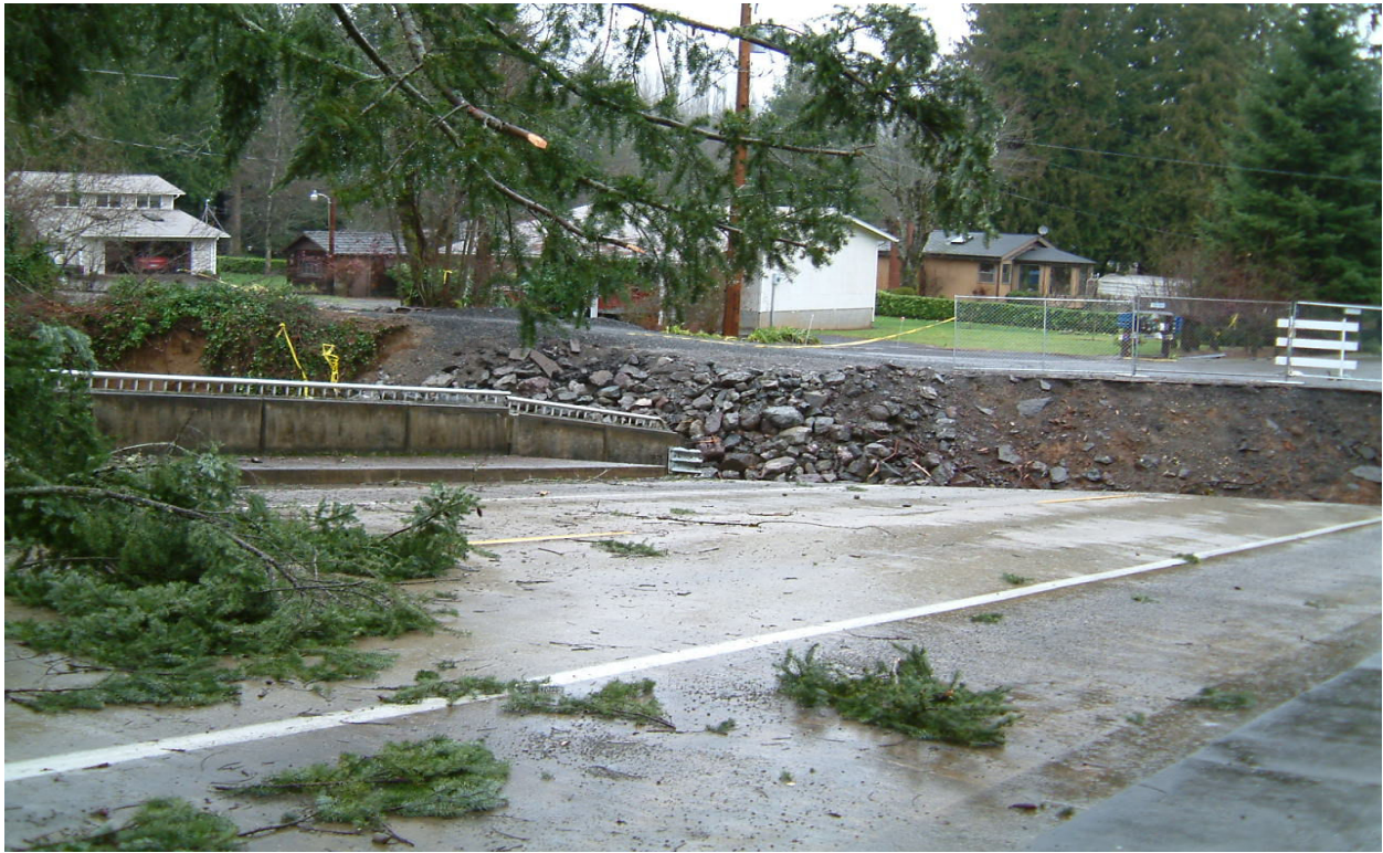
Kitsap County's Chico Way Bridge was wiped out when the north abutment was undermined and collapsed.
