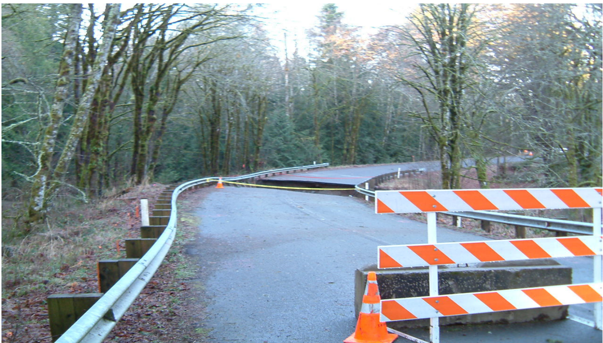
Thurston County suffered severe washouts including the loss of twin multiplate culverts on Cedar Flats Road.
