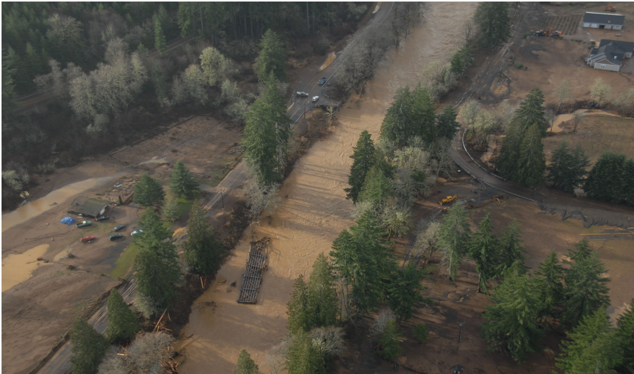
Lewis County's Meskill Bridge across the Chehalis River was obliterated during the December 2007 winter storm and subsequent flooding.
